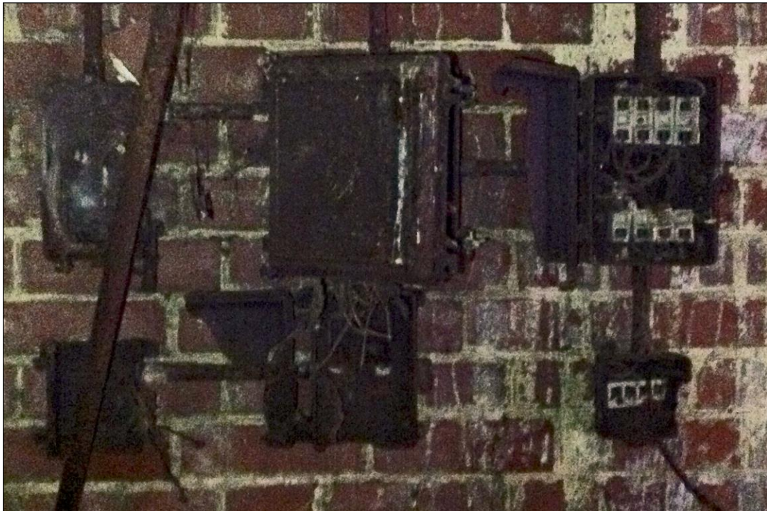
Plate 129: Remains of the electrical switching gear.
