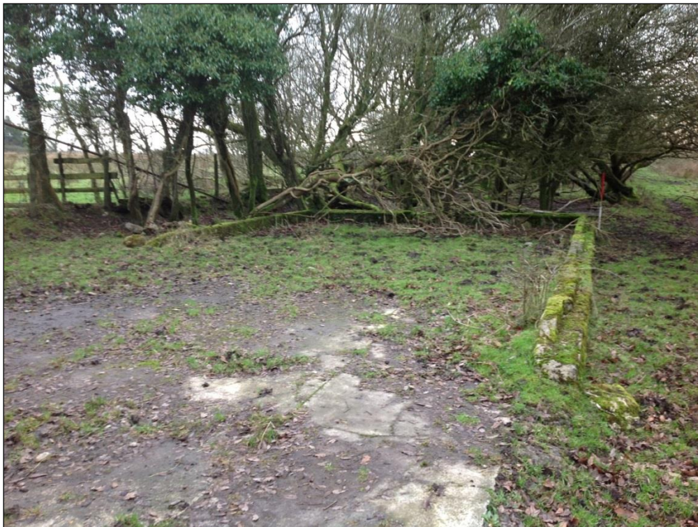
Plate 45: The heavily damaged remains of PRN 07852w.
