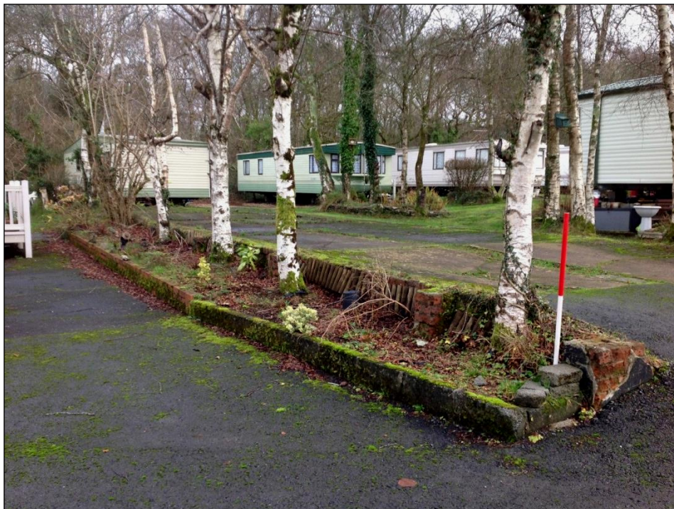
Plate 27: View along the remains of the Institute Buildings west wall
