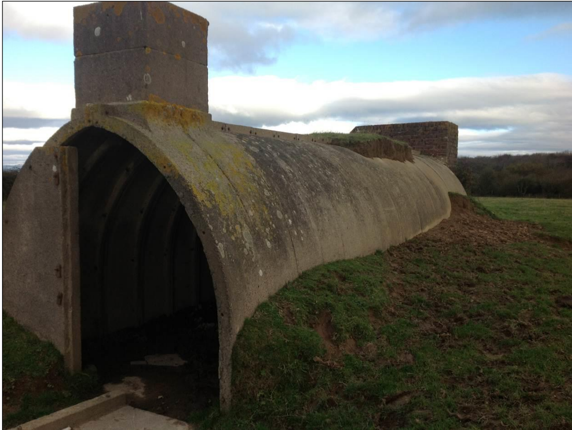
Plate 104: The protective earthen mound surrounding PRN 04444s has been eroded to reveal the construction beneath.
