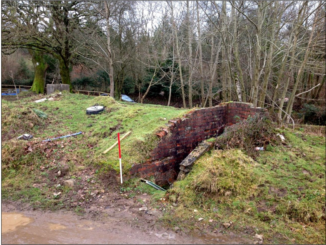
Plate 43: Heavily damaged exterior of the southern Stanton shelter
